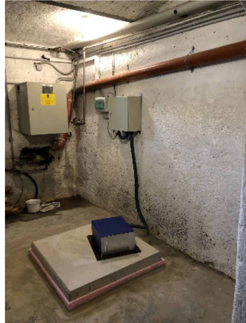
typical strong-motion installation
