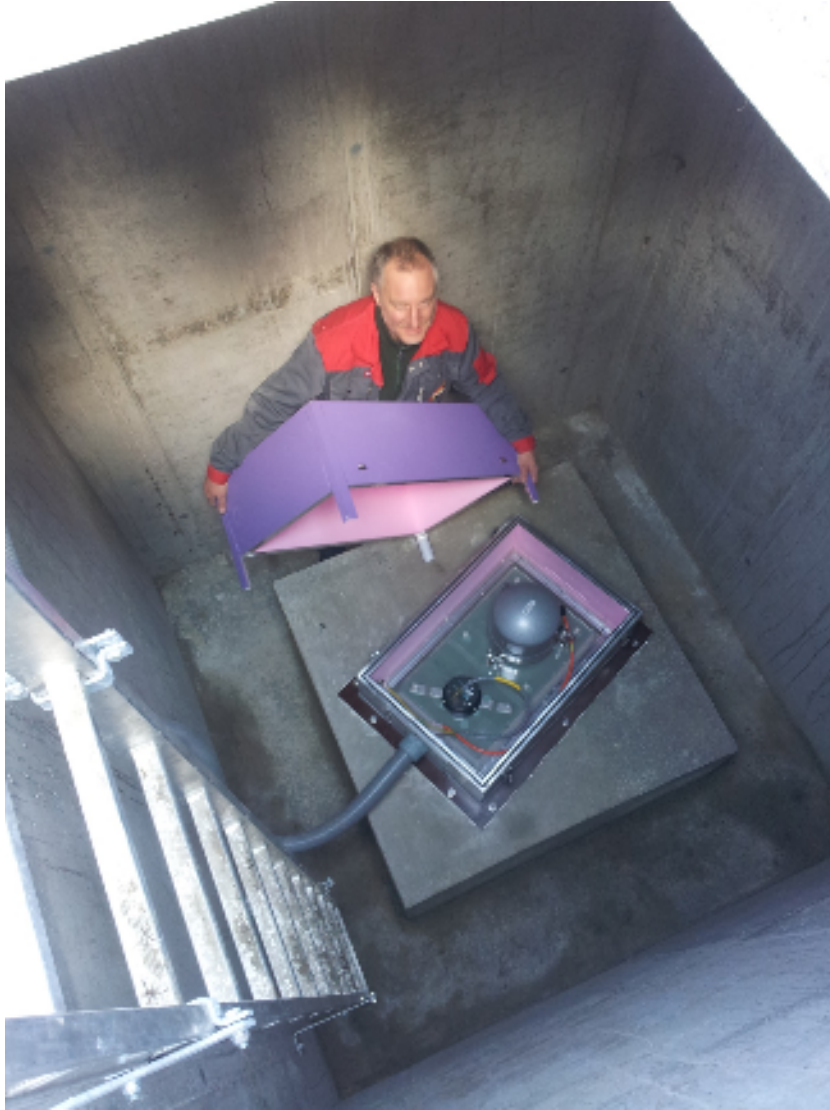
typical broadband installation
