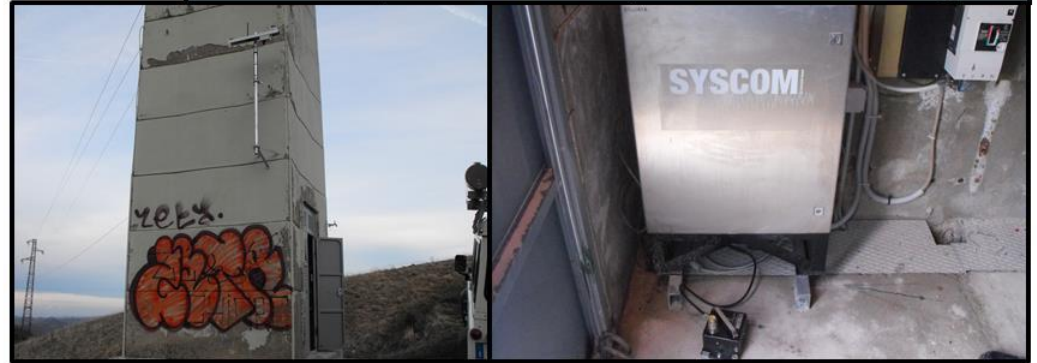
RQT - Arquata del Tronto (inside ENEL's building)
