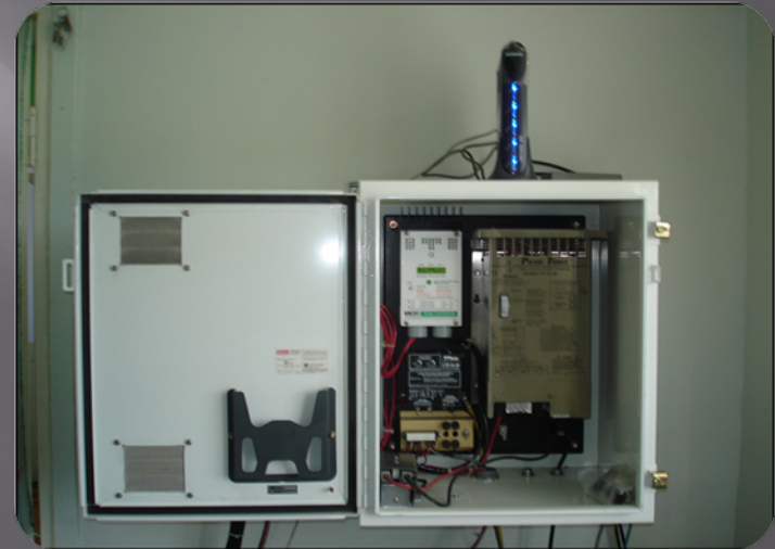
Main power control and management unit
