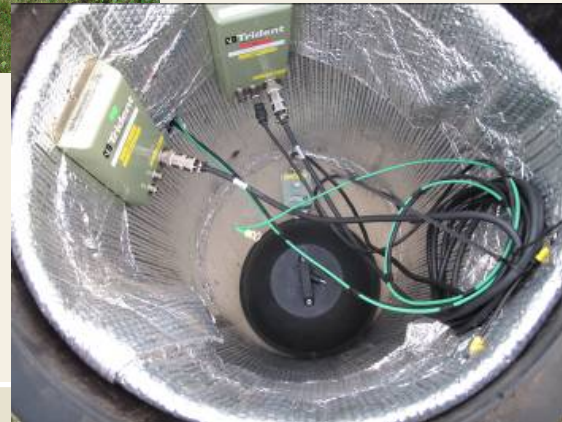
Val-des-Bois real-time station, installed July 24, 2010
