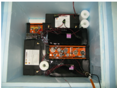
Electronics were stored in insulated boxes
