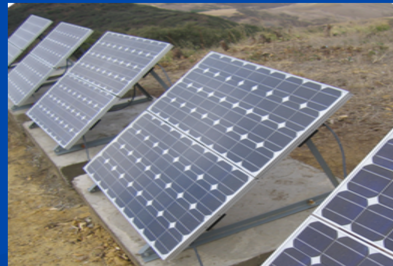
DC Power (Solar Panel)
