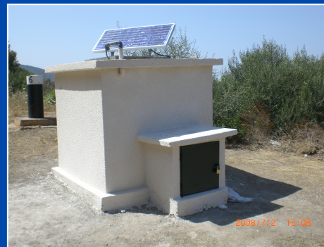
SP Stations in operation
