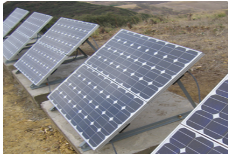
DC Power (Solar Panel)
