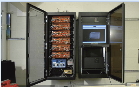
The SMS provides real-time evaluation of the building response based on pre-engineered performance limits. (The OASIS system by Kinometrics is shown above.)
